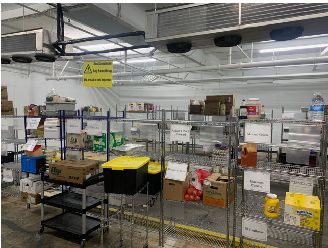
Figure 12. Chef Jeff Project Kitchen, Las Vegas Nevada
